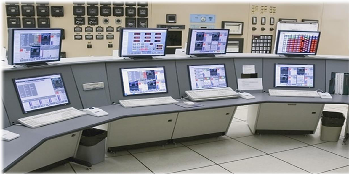
Fig 3.1 SCADA control room
