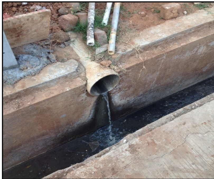
Fig. 1.06. Outlet of kitchen waste
