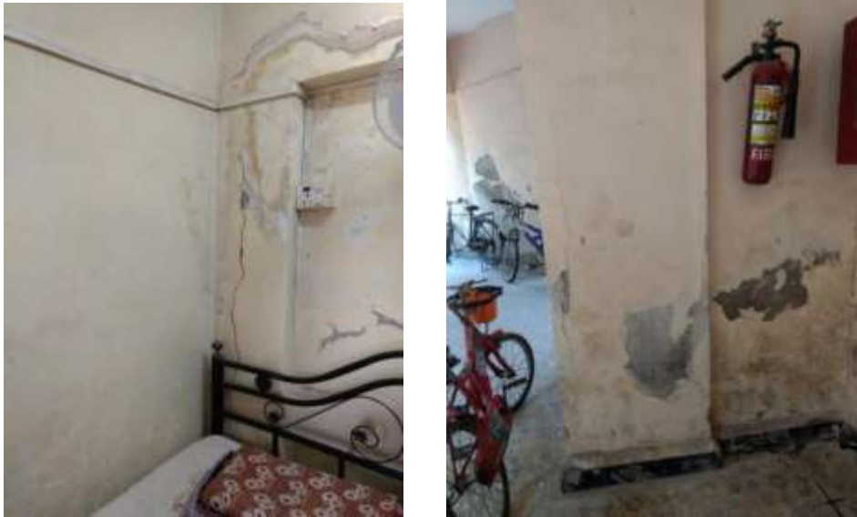
MINOR CRACKS IN COLUMN
