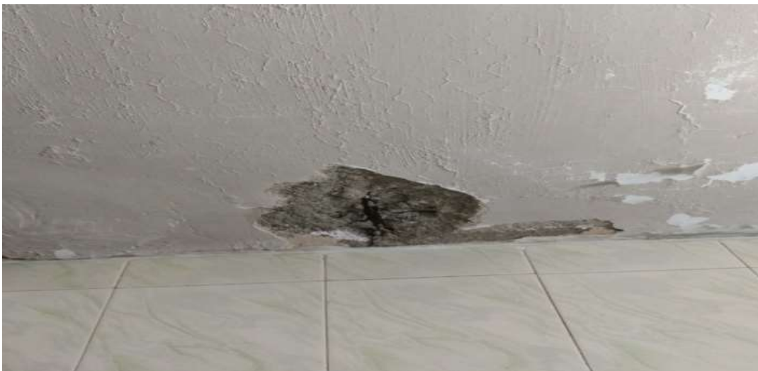
SPALLING OF SLAB CONCRETE
