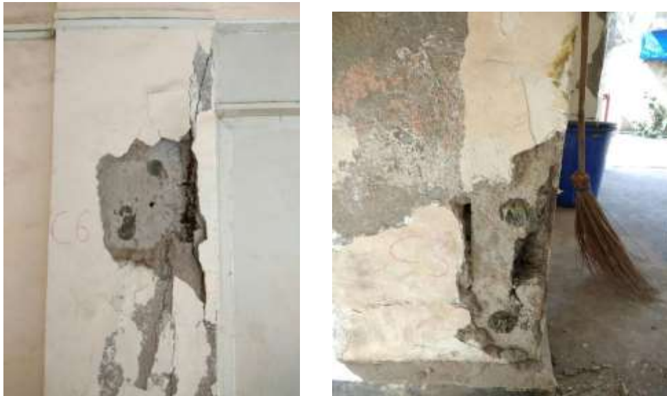
LARGE CRACKS IN COLUMN (GROUND FLOOR)
