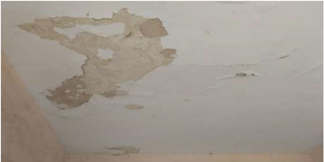
SLAB AT THE ENTRANCE ( HOLLOW WITH VERY LOW UPV VALUE)
