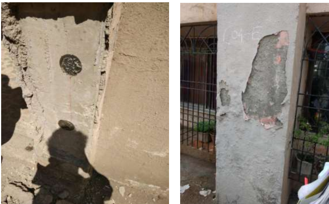
DETERIORATION OF PLASTER
