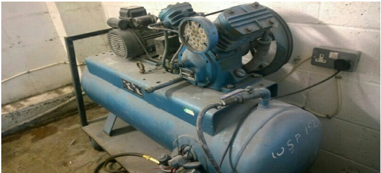
Fig no -3.7 COMPRESSOR .
