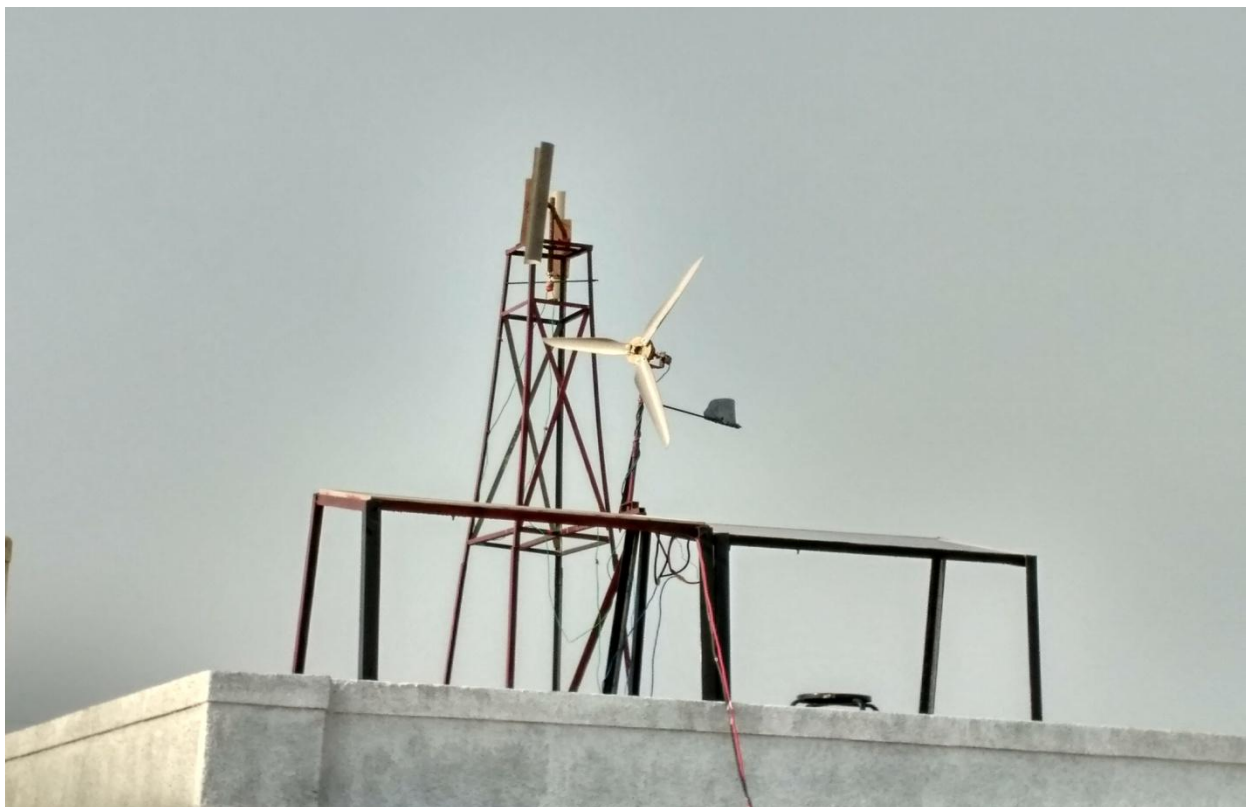
Fig.5.21 Actual setup of Combined System
