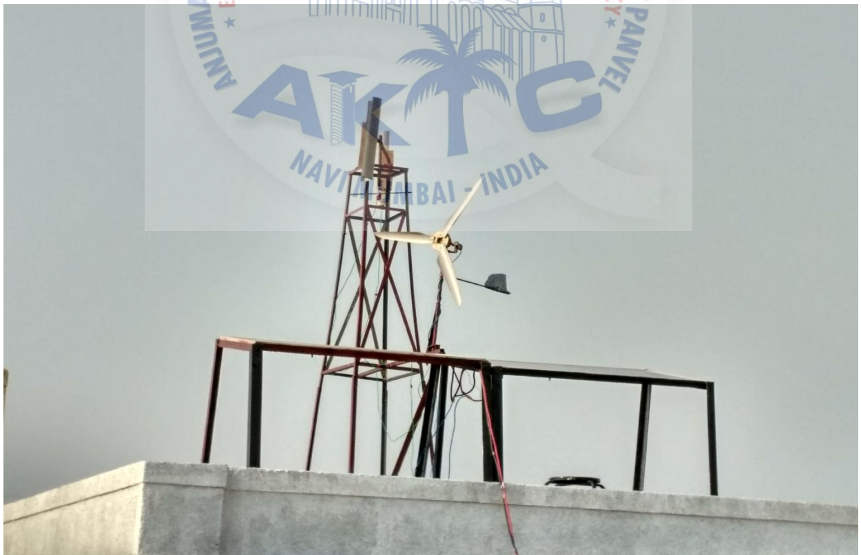
Fig.5.21 Actual setup of Combined System
