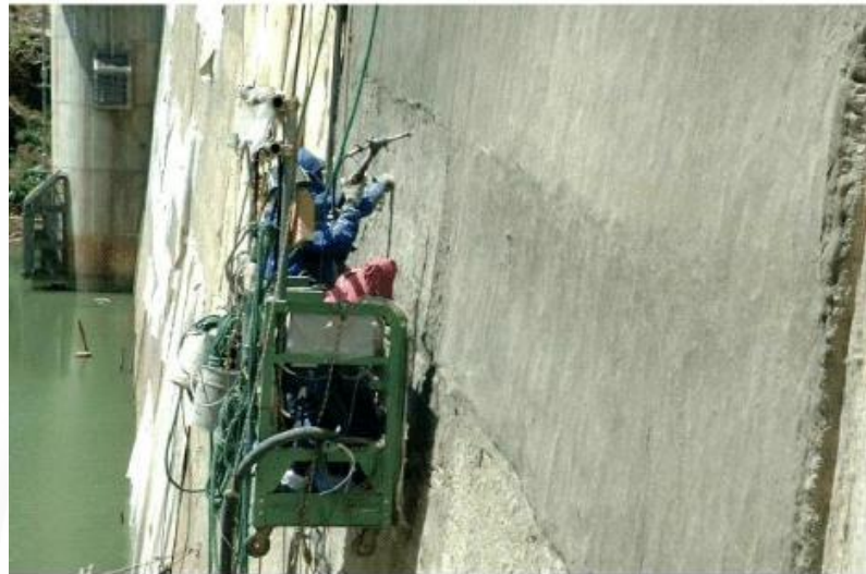
Figure 1. 2: Repair of Mitaka Dam by spraying water-tight ECC layer (Kunieda and Rokugo, 2006)
