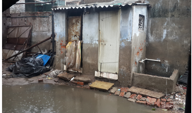
Figure1. 14 Toilets are improper
