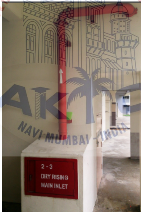
Image showing Dry Riser
