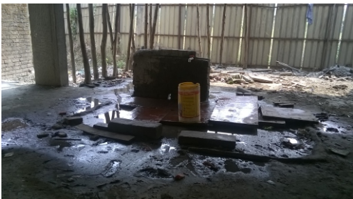
OPEN BATHING AREA. WATER IS DRAINED INTO ADJACENT SITE.
