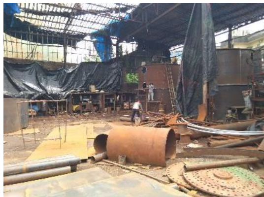
Fig. 4.4. POOR MATERIAL HANDLING.
