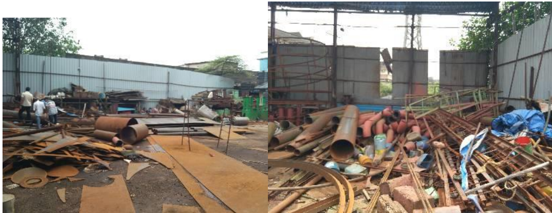
Fig. 4.2. IMPROPER UTILIZATION OF WORKSPACE AREA.
