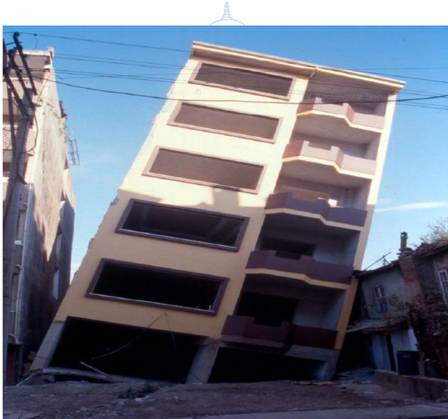
Fig .10. Failure Caused due to excessive Drift [1]
