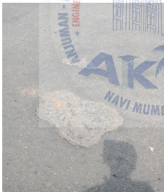
Fig 4.5: Depressions on selected pavement surface
