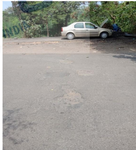
Fig 4.2: Ravelling on selected pavement surface
