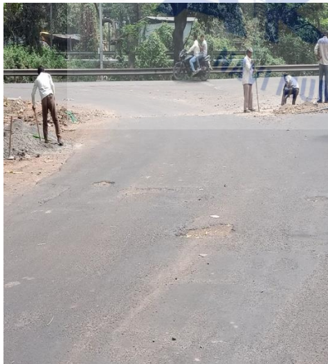
Fig 4.1: Potholes on selected pavement surface
