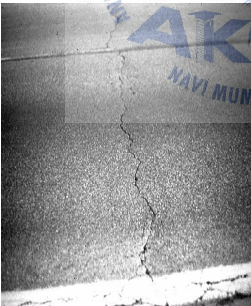
Fig 3.5: Low Severity Transverse Crack
