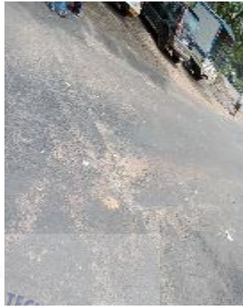
Fig 4.4: Edge cracking on selected pavement surface
