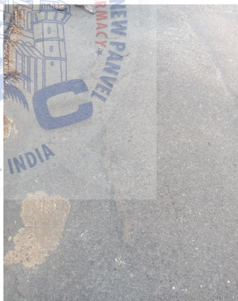
Fig 4.6: Longitudinal cracking on selected pavement surface
