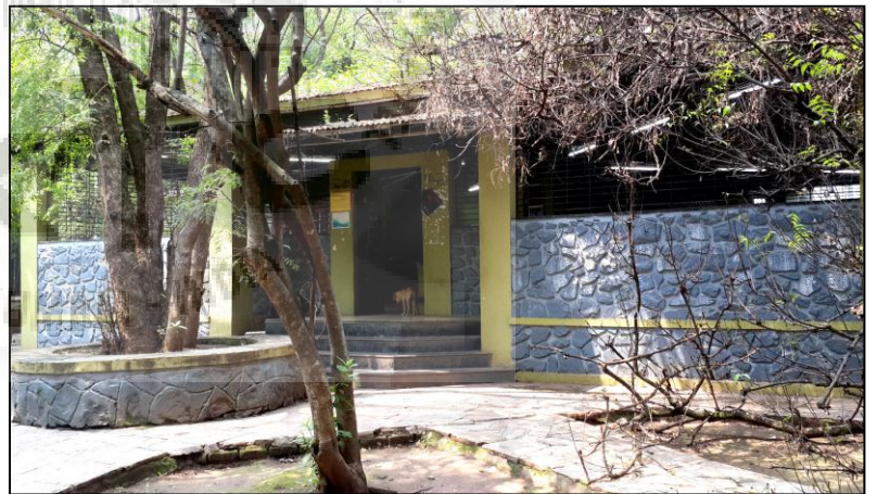
Figure 10. Images showing condition of structure
