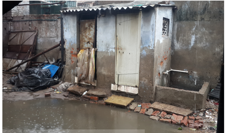
Figure1. 14 Toilets are improper
