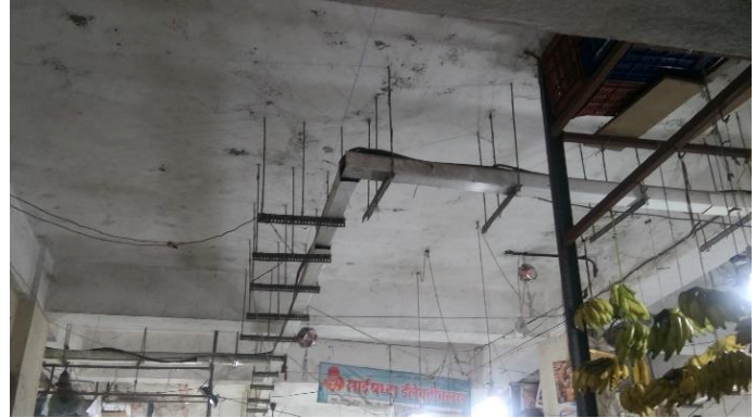
View of ceiling showing main electrical line running
