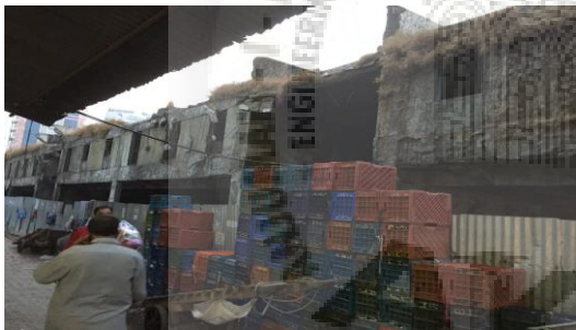
Main structure is in dilapidated condition
