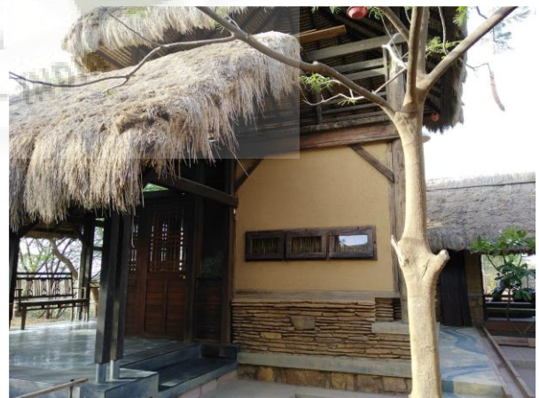
Image showing the roofing made from thatch. Which is supported on timber and steel members.
