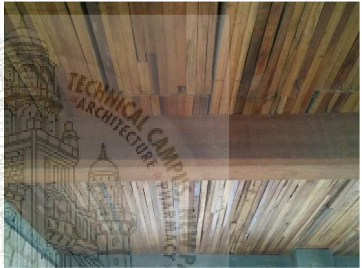
Image showing the roofing made from waste timber, which is collected from old ships from mandhvi port
