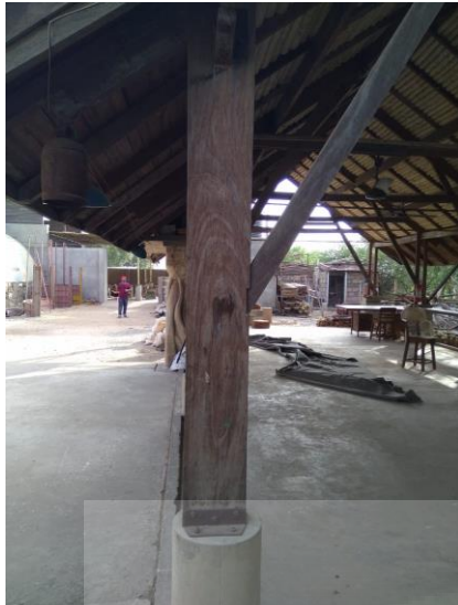
Image showing the column made from wooden log used as a structural member joined with concrete base
