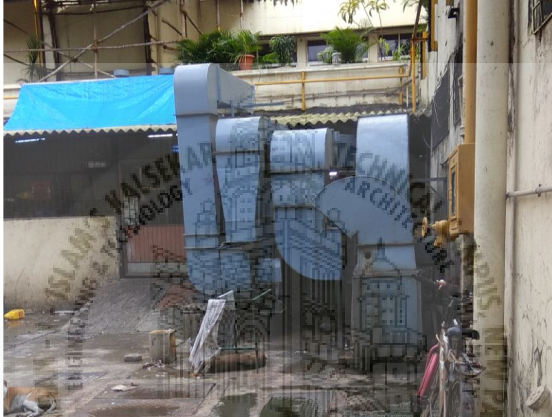
Ducts behind the restaurant wall
