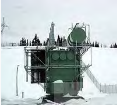
Transformer at the Limestone Generating Station in Manitoba, Canada
