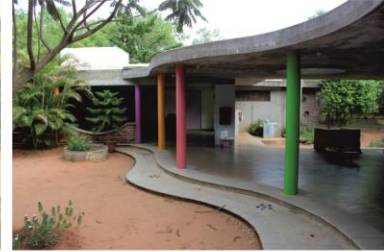
C2 Figure No:16 ORGANIC FORMED CORRIDOR BETWEEN CLASSROOMS AND PLAY AREA- STEPS
