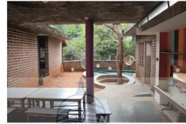
C2 Figure No:18 TRANSITION AREA BETWEEN TWO SPACES-WASHBASIN AREA AND KITCHEN CLEANING AREA
