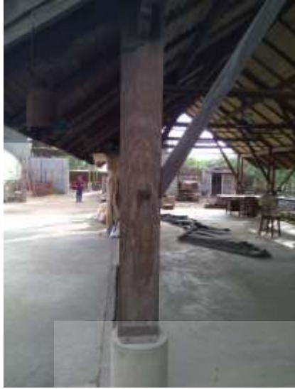
Figure 30: Column made from wooden log used as a structural member joined with concrete base
