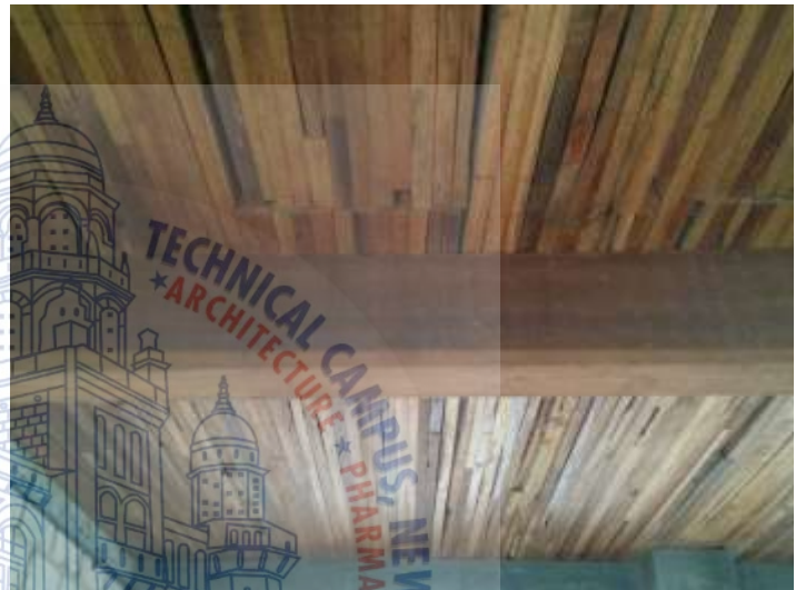
Figure 21: The roofing made from waste timber, which is collected from old ships from mandhvi port
