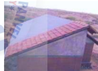
Figure 44: the gabled roof construction with layer of 30mm perlite filling and Mangalore tiles as a final finish
