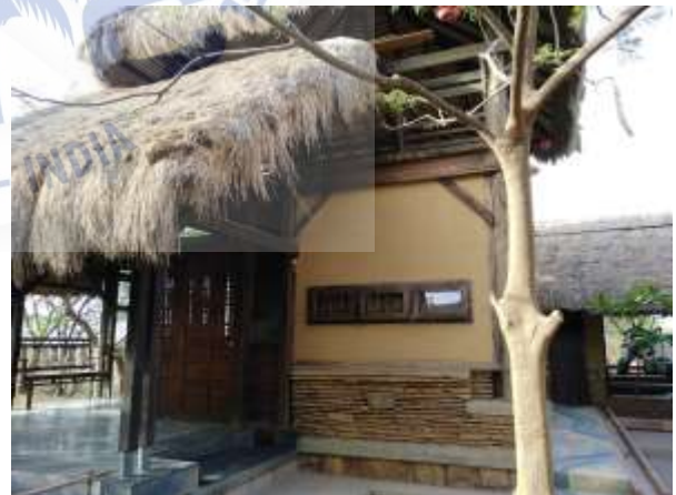
Figure 23: Roofing made from thatch. Which is supported on timber and steel members.
