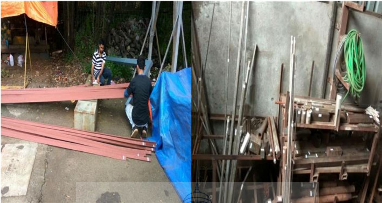
Fig. 1.1 Poor utilization of space
