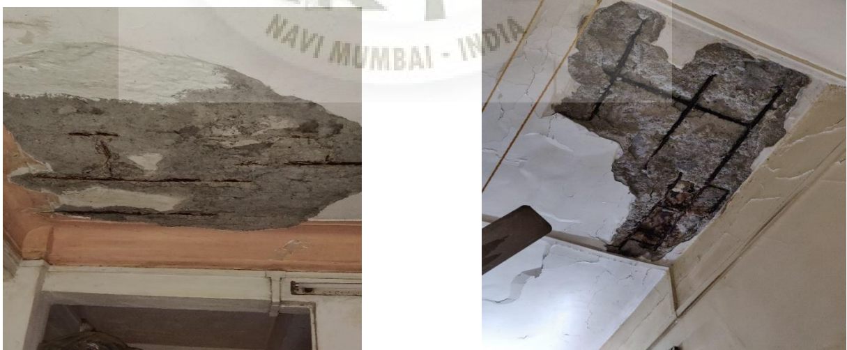
fig no. 5.5 deterioration of plaster
