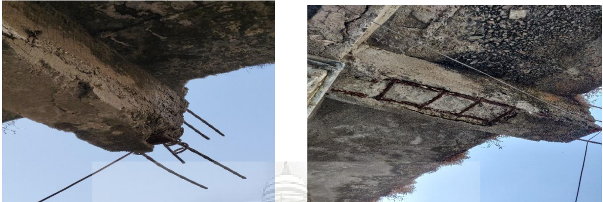
fig no. 5.6 Beams open to atmosphere with visible reinforcement
