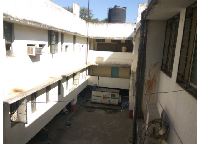
Figure 31 : - Services lines are used in courtyard
