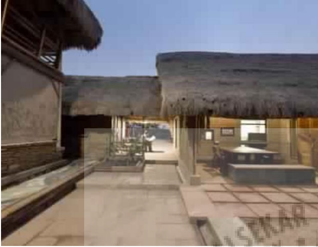
Image showing the roofing made out of thatch which is supported on timber and steel members
