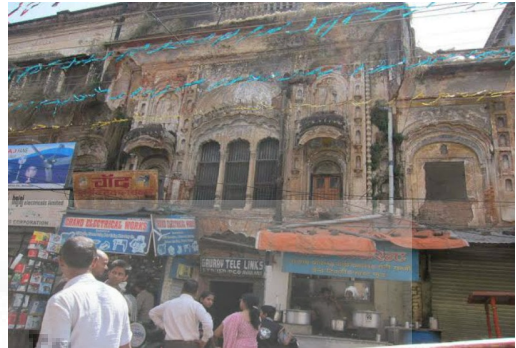
Fig.5.1.4(A) Image Showing Poor Condition Of Buildings
