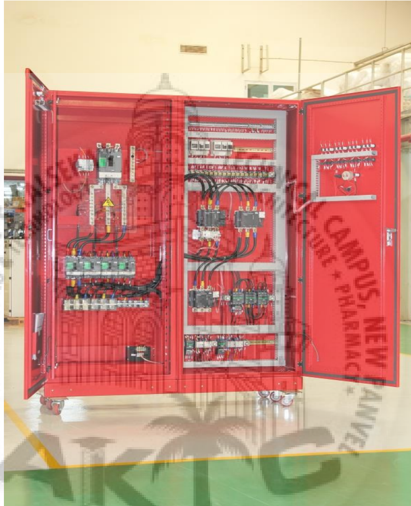
Figure 6.1 Fire Control Panel
