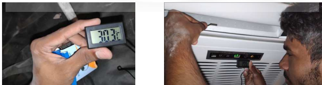
Fig.4.48. Checking for working of system
