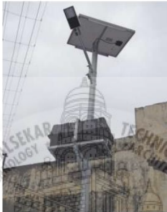
3.1 actual photo of street solar light system
