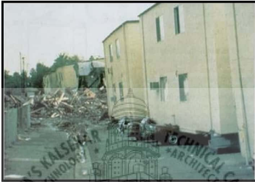
Figure: 3.8 Total collapse of Soft Storeyed at Open Garage at the Ground Floor of the apartment Building in Northridge Earthquake (cars parked at the garage level seen to be crushed)
