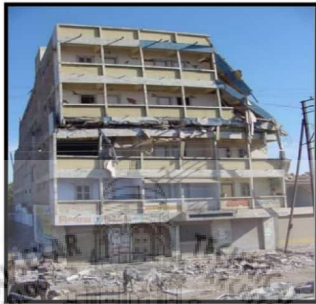
Figure 3.10: Collapse of Soft Middle Storey in a Building at Bhuj
