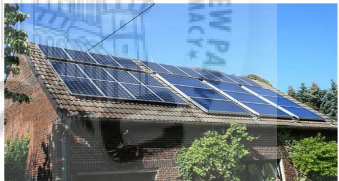
fig 3.2-Solar PV panel at rooftop
