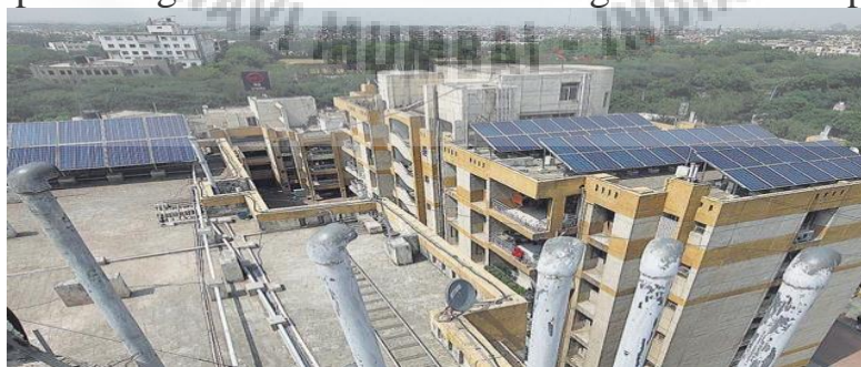
Figure 3.3-Solar PV panel at building terrace
