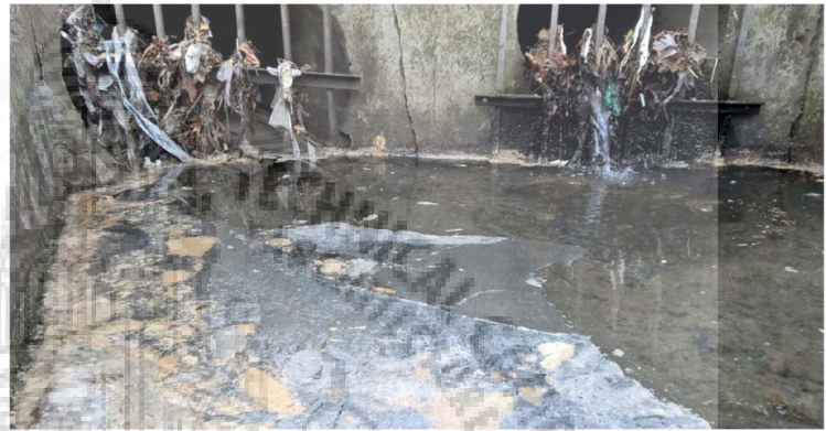
Water stagnation and water pollution problem
