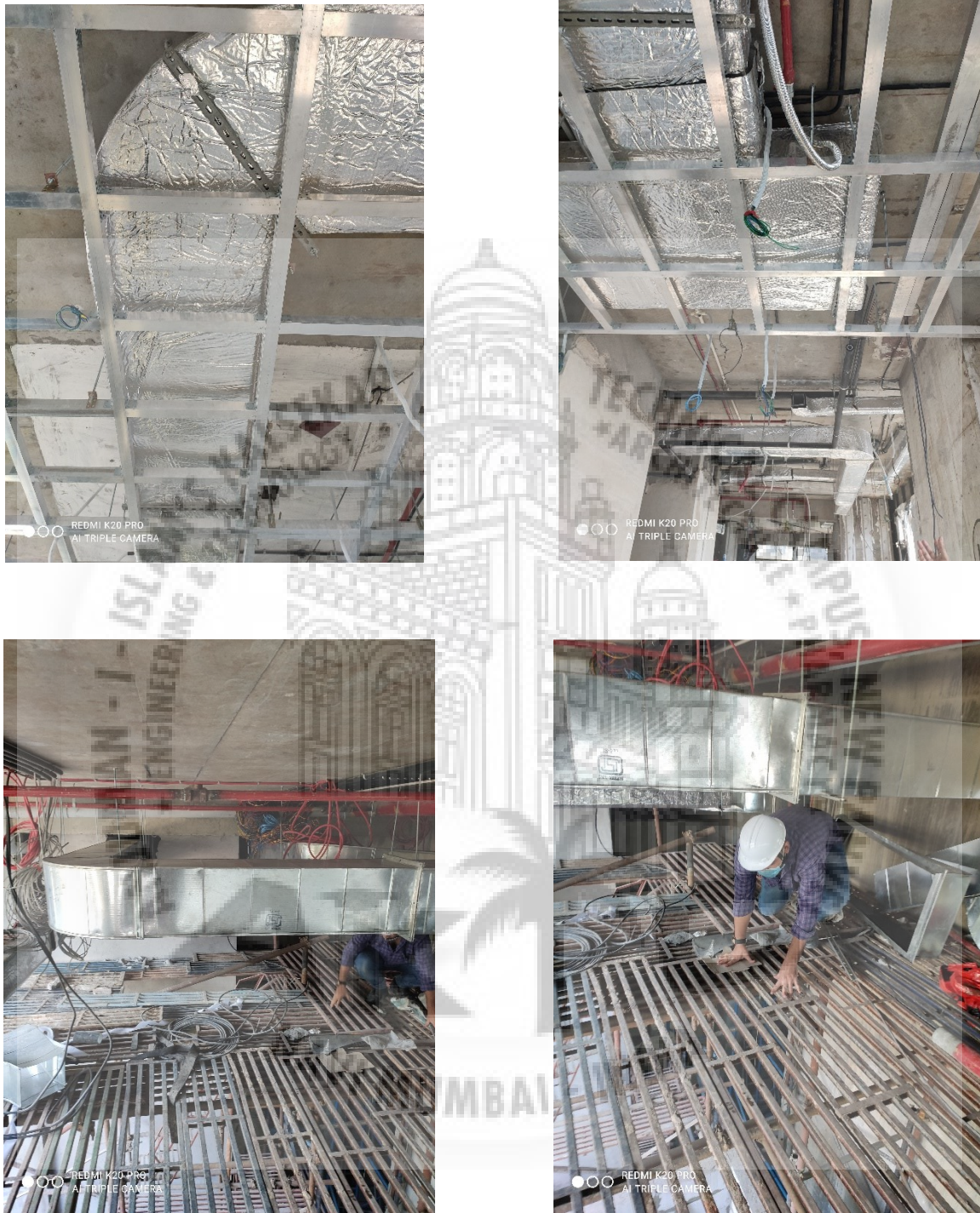
Figure 8-5. Ducting in Living Room.
