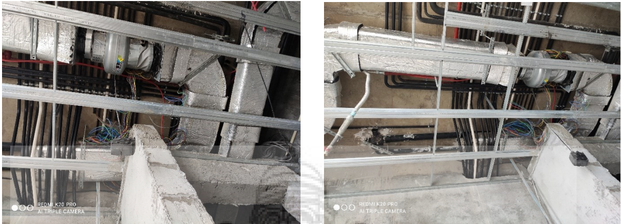
Figure 8-7. Inline fan in Kitchen for Exhaust (1400CFM).
