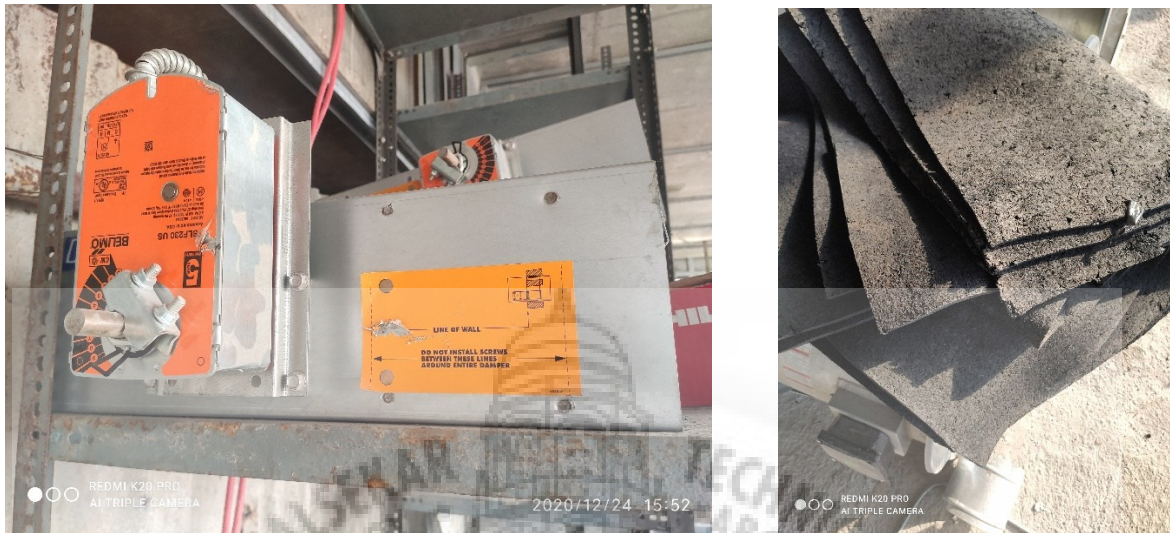
Figure 8-9. Smoke Fire Damper & Arma Sound.
