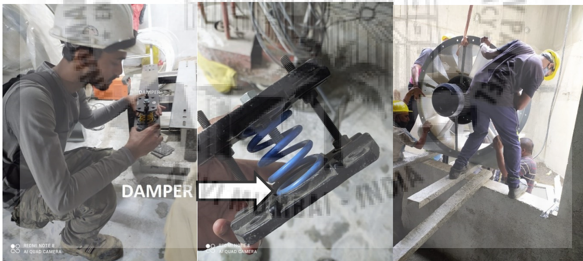
Figure 8-18. Damper & Turbo fan (36000 CFM) for Fresh air.
