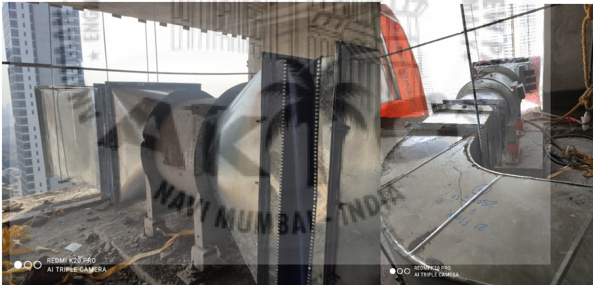
Figure 8-8. Inline fan for fresh air (4000 CFM).
