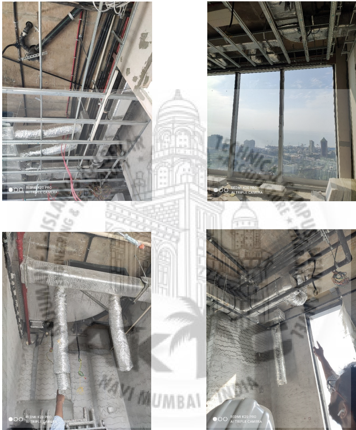
Figure 8-6. Ducting in Bedroom & Bathroom.
