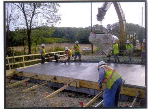
Figure 5: Internally Cured Concrete Bridge Deck being Cast Near Bloomington, IN (Di Bella, Schlitter, & Weiss, 2010)
