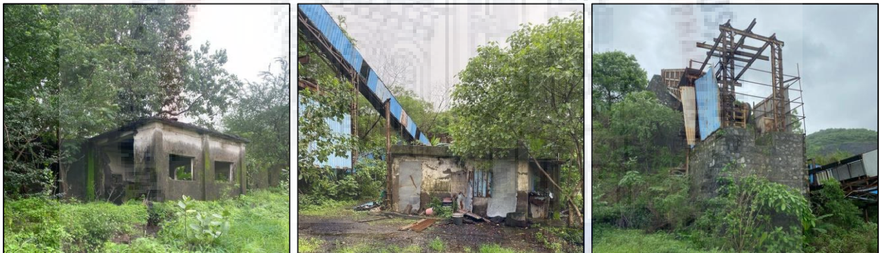
(Figure 125, Dilapidated & abandoned structures)
